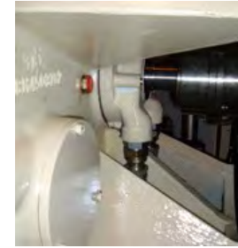
Fig. 24: Main oil pump
