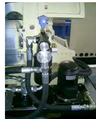
Fig. 23: Multi-function device & pre/post lube oil pump
