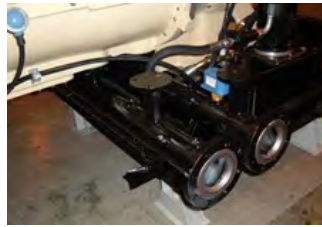
Fig. 17: Cooling water manifold
